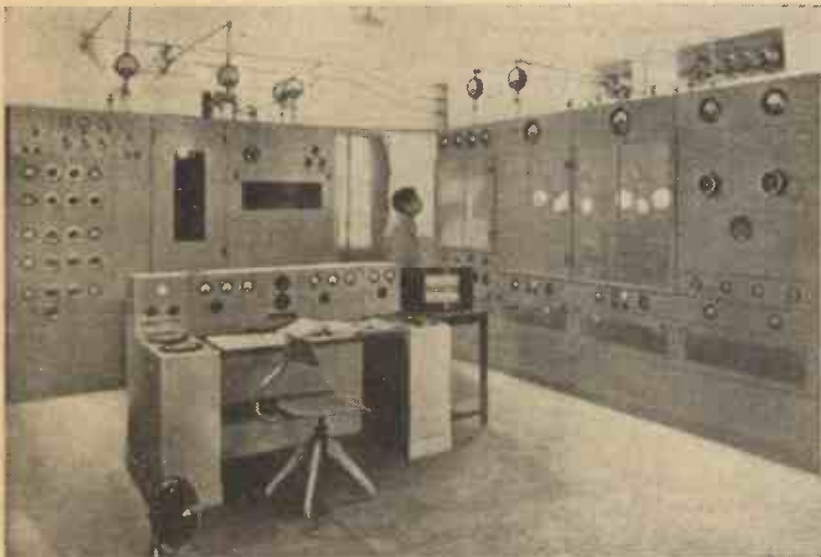
The task of changing to any desired wavelength between 25 and 90 metres can be carried out in less than ten minutes with the Philips 10-kW short-wave transmitters in use.
